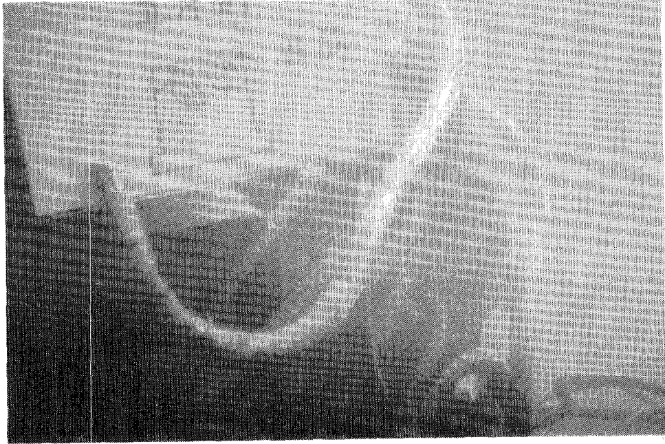
Photo-9 Underwater View of Exposed Ferro-concrete Bars of Reinforcement of a Broken Caisson No. 20. (Courtesy to Nishimatsu Construction Co. Ltd.).
