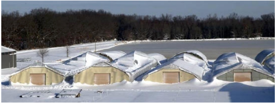
Collapsed greenhouses just off Interstate 24 in Paducah. The weight of a record-breaking snowfall proved too much for several structures across western Kentucky. The total snowfall of 14.2 inches at Paducah set a 24-hour snowfall record. Photo courtesy of Beau Dodson.
