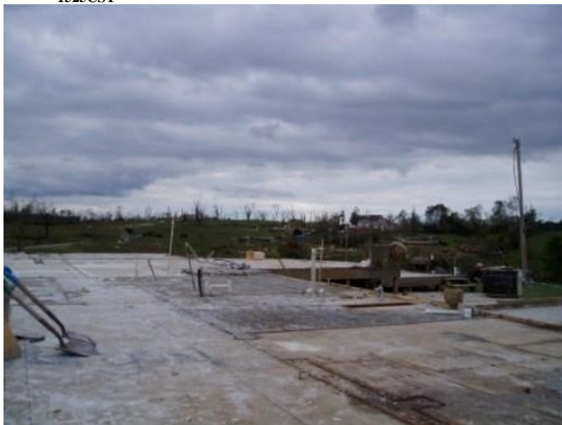
House swept clean off foundation near Crosstown.
