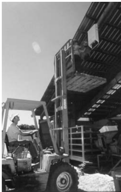
Photo 3. Rachael Long, farm advisor with the University of California (Yolo County) Cooperative Extension, installs two wooden bat houses on a pole barn at Ferrari Farms, near Linden, CA.
