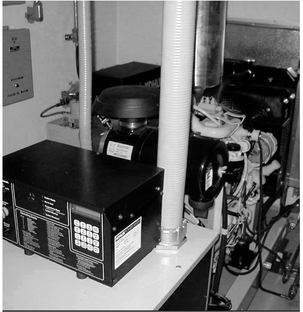
Figure 14: Aviation Services: FAA-Provided Electrical Power Generator in Honolulu, Hawaii, Headed for the FSM and the RMI
