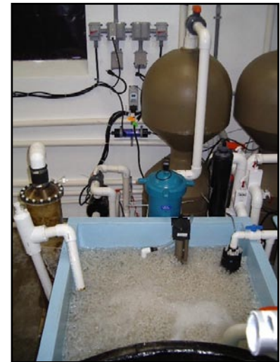
Fig. 1. RAS water treatment
