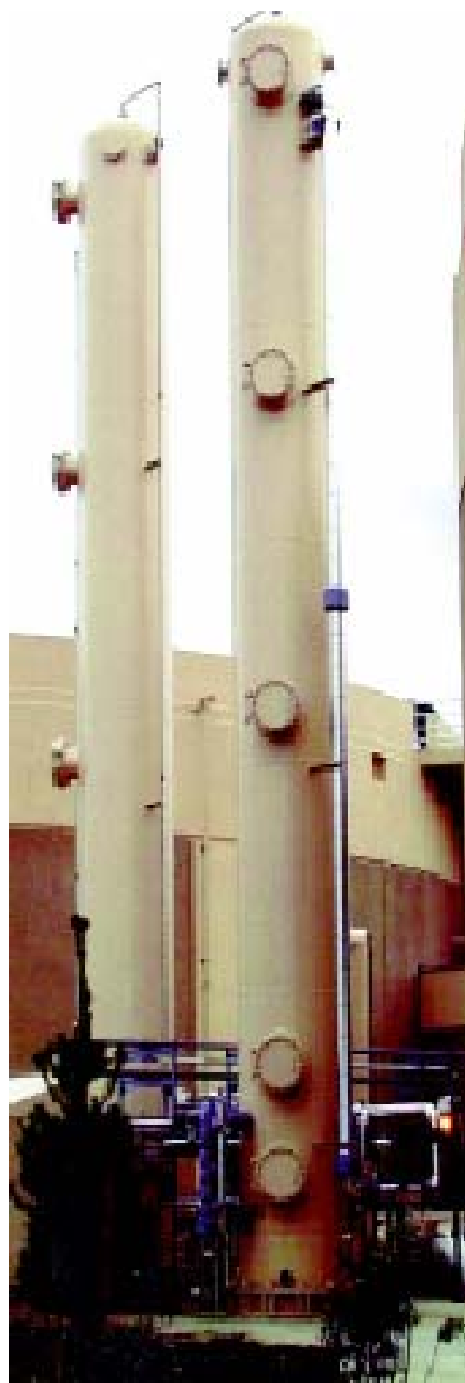
Figure 3-1 Carbon dioxide absorption towers at the King County South Wastewater Treatment Plant
