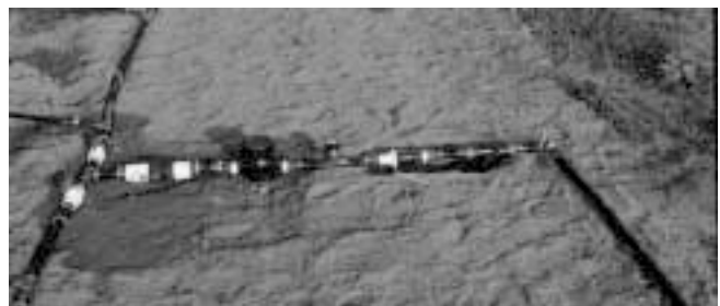
Irrigation mainline with screen filter, pressure regulator, pressure gauge, and water meter connected to sub-main
