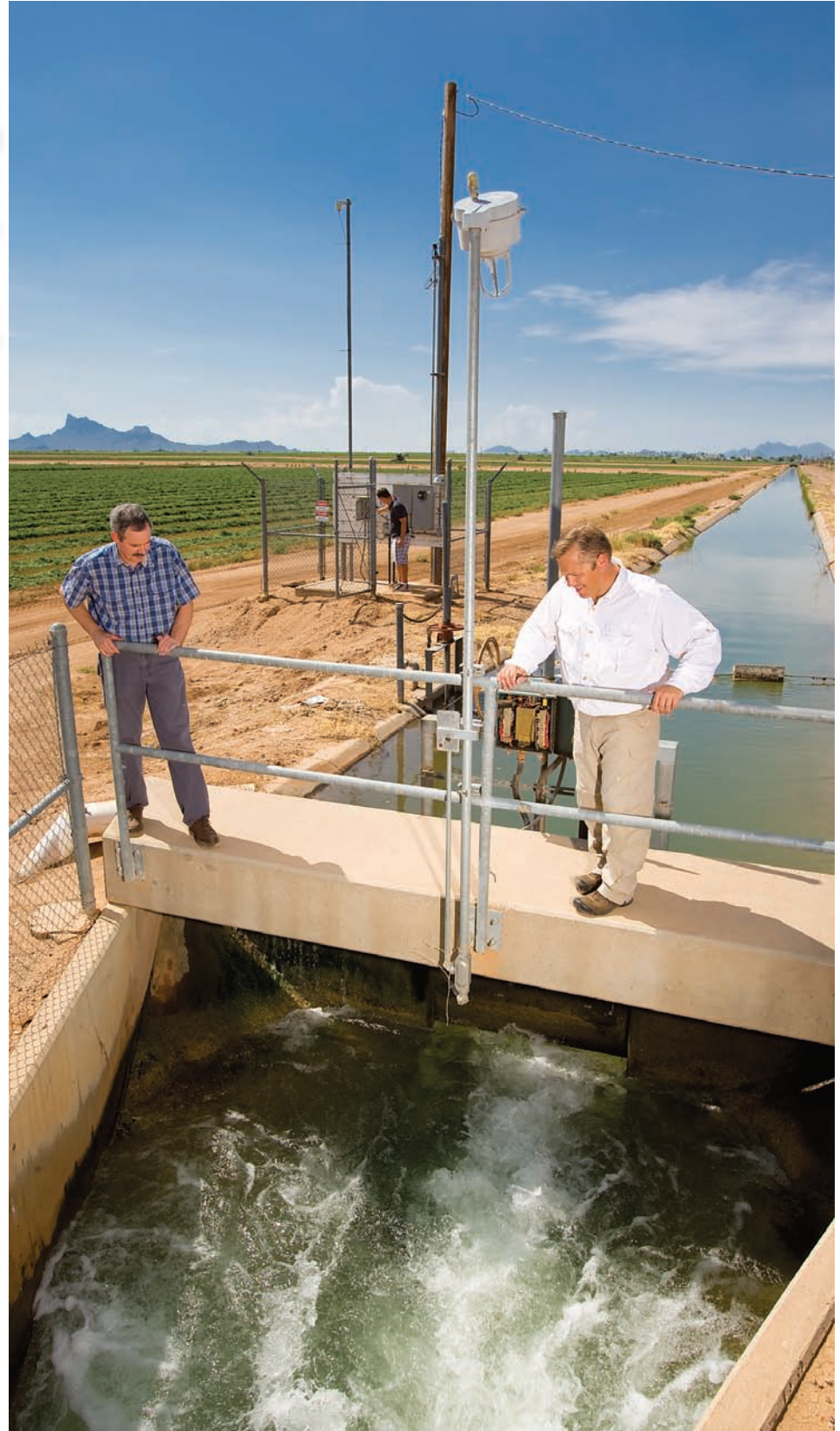
At the Central Arizona Irrigation and Drainage District, hydraulic engineer Bert Clemmens (left) and electrical engineer Bob Strand assess the automatic control of one of the many hydraulic gates operated by ARS-developed software while student Matt Robbins (background) checks the communications.
