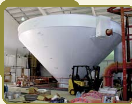
Sandoval- The treatment unit at Gateway Regional Water Company's water treatment plant is part of the system Rural Development supported with substantial technical and financial assistance. It will be operational in 2008 and supply nine rural entities serving 20,000 people in four counties. Years of commitment, coordination and infrastructure development were needed to complete the Gateway project.
