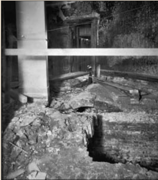
The stone floor in today's "small Senate rotunda" was blown away by the force of the gas explosion that rocked the Capitol on November 6, 1898.
