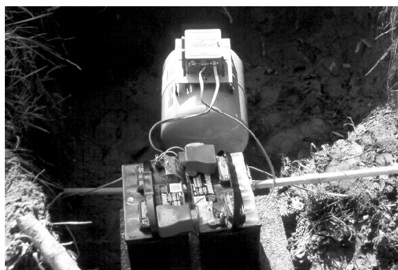
Figure 8. Pressure Tank and Batteries
