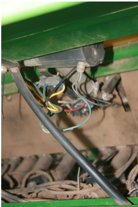
This is a photo of the linear actuator that opens and closes the door on the air seeder. The door was present on the air seeder when it was purchased.
