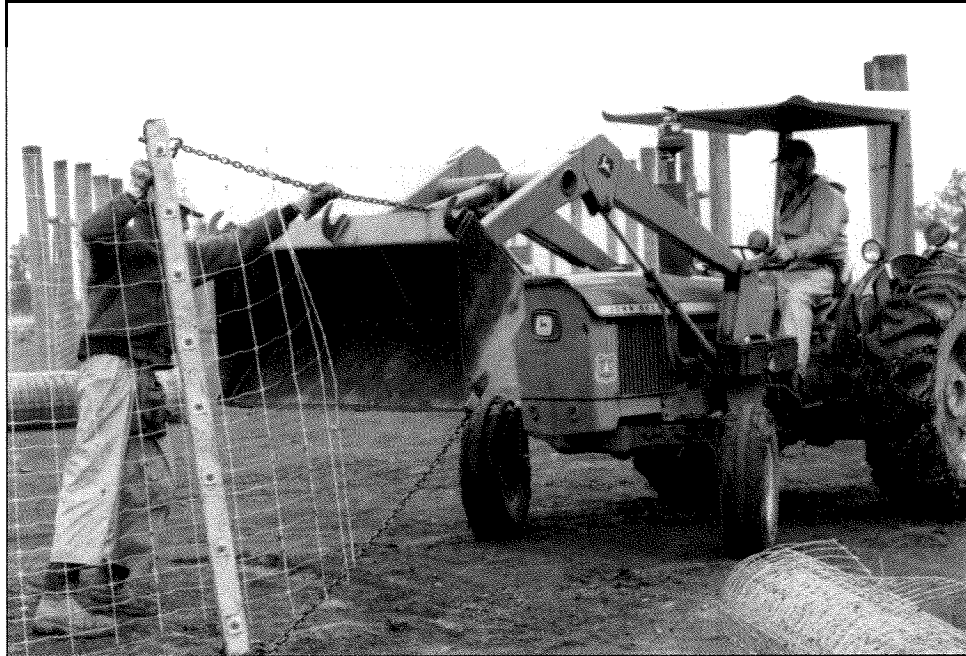
Figure 1 -Construction of the game-proof fence at the Starkey Experimental Forest and Range enclosed the native herds of mule deer and elk, which became the experimental population.
