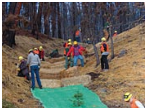
BIRT volunteers construct a straw check dam, spread straw mulch, and use erosion mats to protect this drainage.
