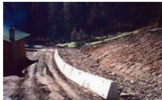
Right: A concrete barrier and rock-lined channel, funded through EWP, were used to protect the Roberts' home on Dickson Creek. In total, EWP funds were used to build 729 feet of concrete barriers.
