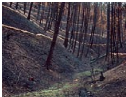
Left: NRCS engineers suggested appropriate erosion control practices for each situation. Here straw wattles were used to stabilize slopes.
