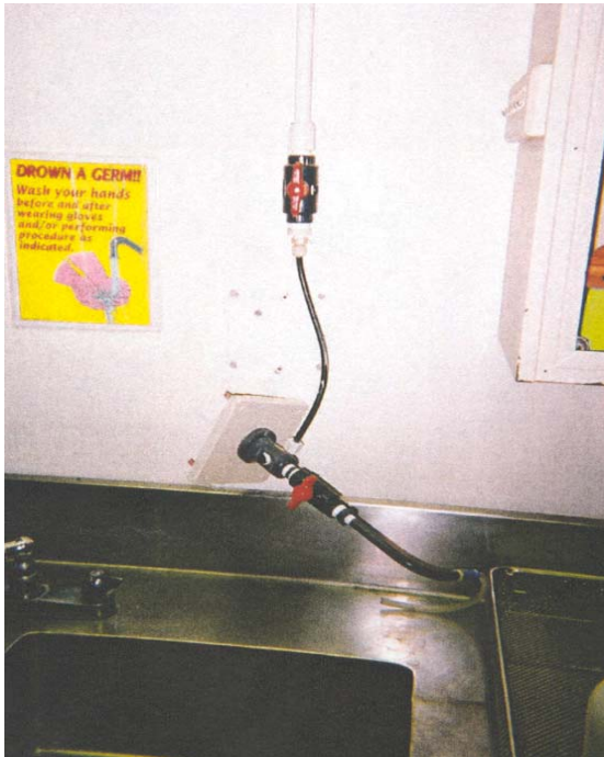
Broken Cleaning Equipment in SPD
