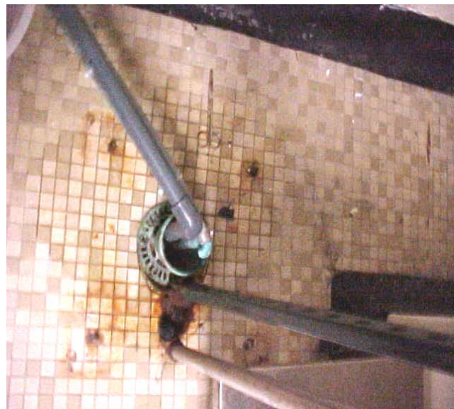
Dirty and Rusty Hemodialysis Drain Area
