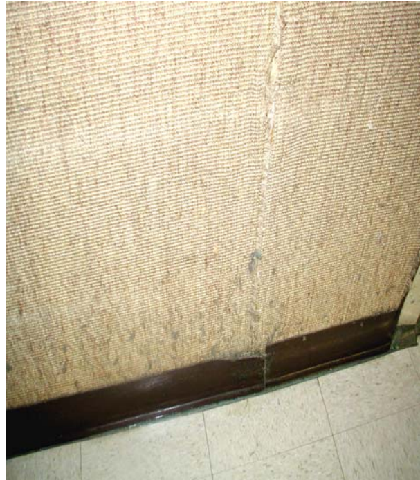
Dirt Accumulation on all Walls in Primary Care
