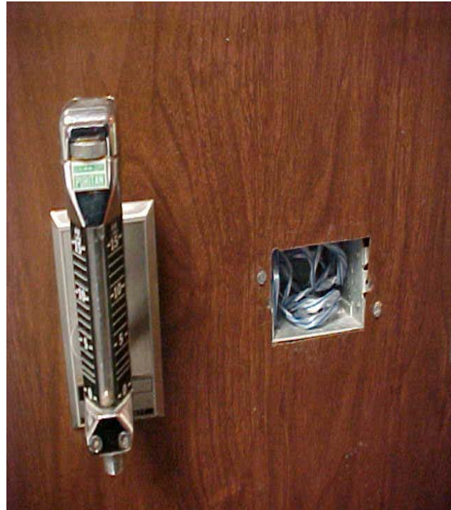
Open Electrical Wiring Near Patient Bed
