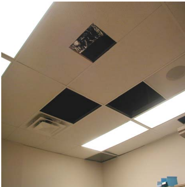
Missing Ceiling Tiles in Primary Care
