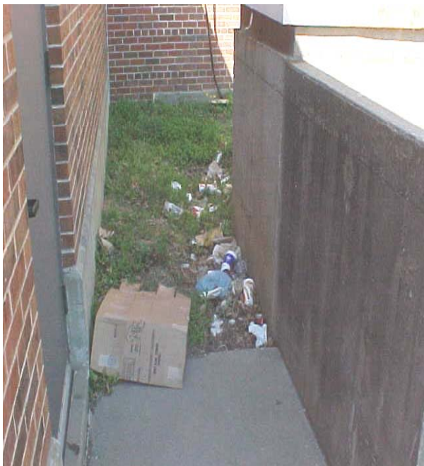
Trash Accumulation Near Back Entrance
