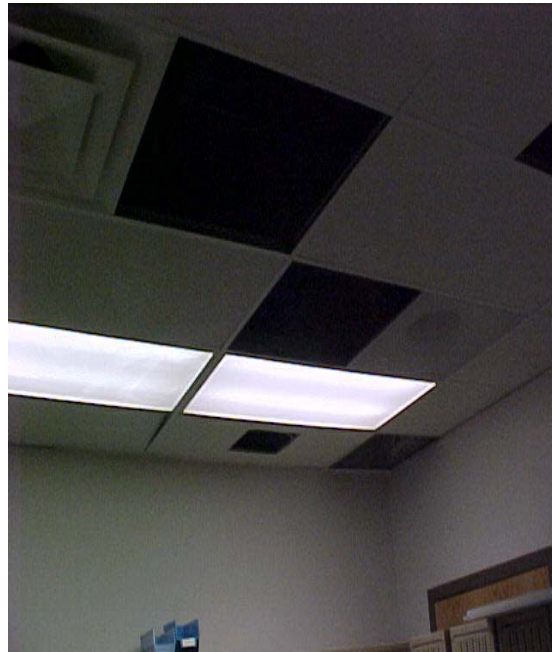
Missing Ceiling Tiles
