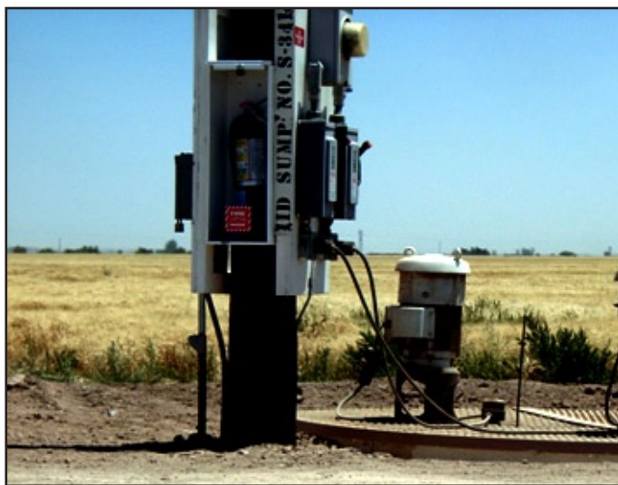
Figure 11 Down Gradient Sump Discharging to Treatment System
