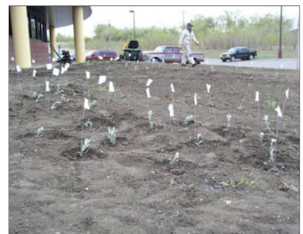
Construction of medicine wheel at Northern Lights Community Center in New Town
