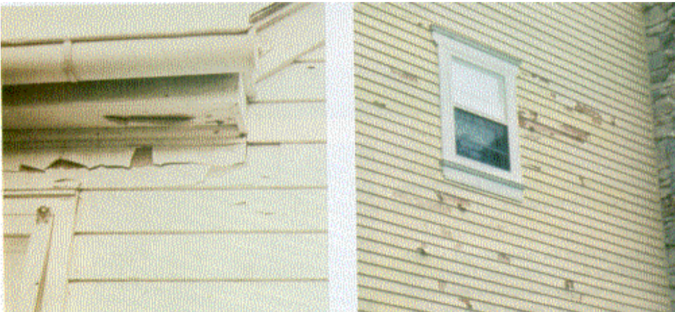
Excess moisture causes peeling paint. Leaking gutters and roofs, ice dams and inadequate overhangs are some of the typical causes of peeling paint.
