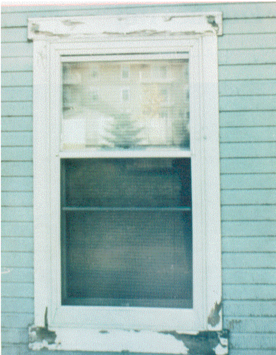
Moisture from the inside will cause peeling paint on the outside. Moisture-laden air escaping from around a leaky window will cause paint to fail at the point of exit.
