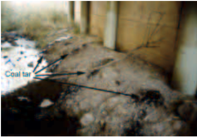
Figure 51—Coal tar deposits in a small stream flowing under an unnamed bridge in Oregon. Coal tar was used to seal cracks in the asphalt covering on this bridge.
