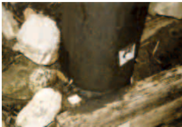
Figure 20—Creosote weeping from pressure-treated piling at Bridge 148.
