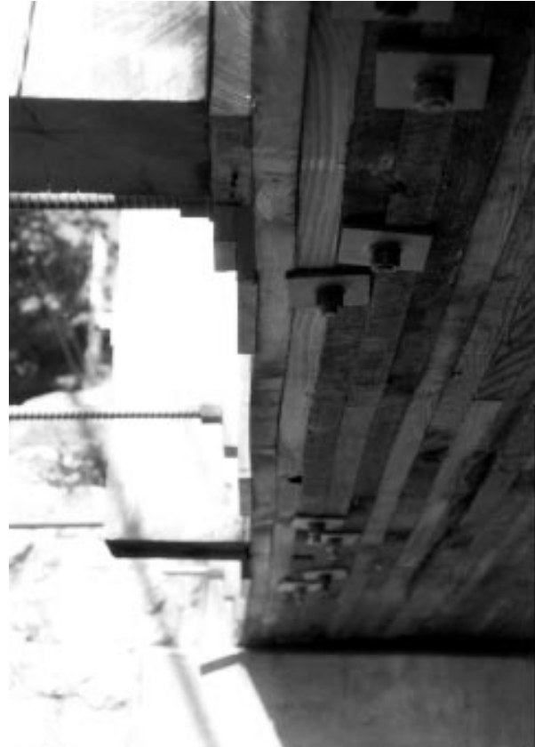
Figure 26—Distorted exterior lumber lamination noted during condition assessment at the time of load test 2.
