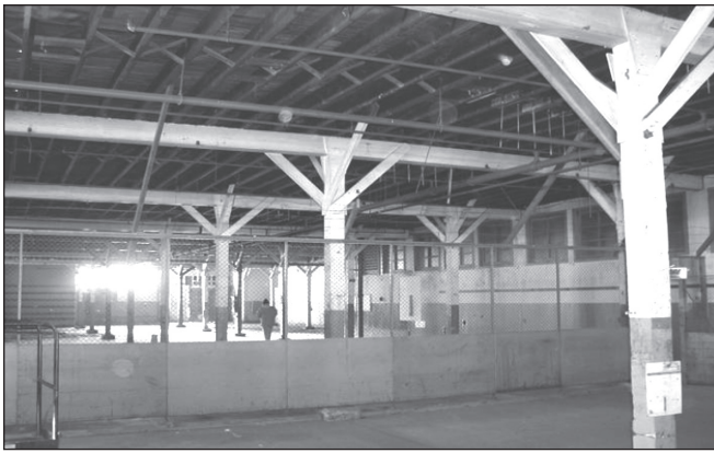
Figure 3—Twin Cities Army Ammunition Plant (TCAAP) warehouse, New Brighton, Minnesota, before deconstruction.
