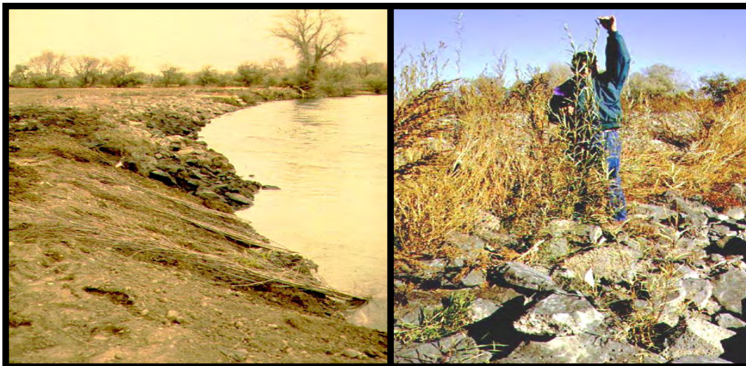
Figures 2 and 3: Vertical bundles are placed on 6 feet centers with the tops 1 foot above the top of the bank and the bottoms touching the bottom of the keyway trench. Four months after planting, the vertical willow bundles have grown approximately 6 feet.
