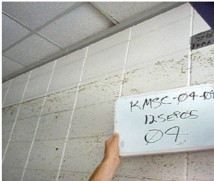
Figure 6 – Interior Mud Line HWM
