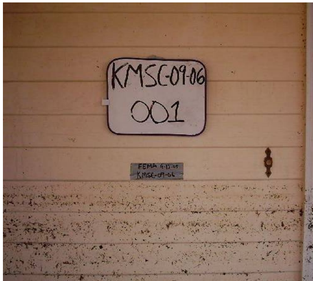
Figure 7 – Exterior Mud Line HWM
