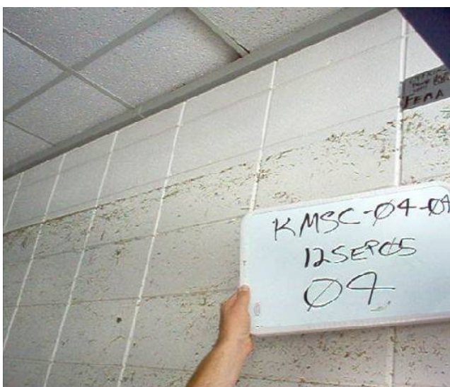
Figure 6 – Interior Mud Line HWM
