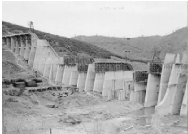
1.14. Photo taken during construction of Stony Gorge Dam, California from downstream side. Note struts between buttresses and sloping slabs on left side of photo.
