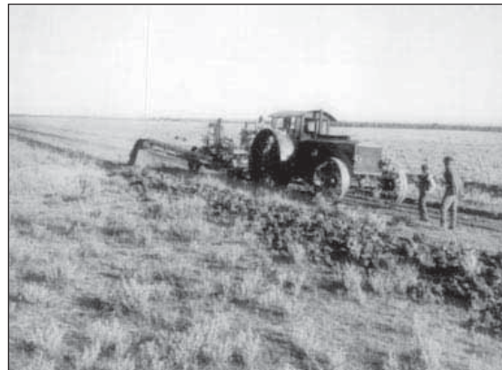
4.1. In October 1913 a Pioneer traction engine pulled an Austin elevating grader digging drainage ditches on the Milk River Project near Malta, Montana.
