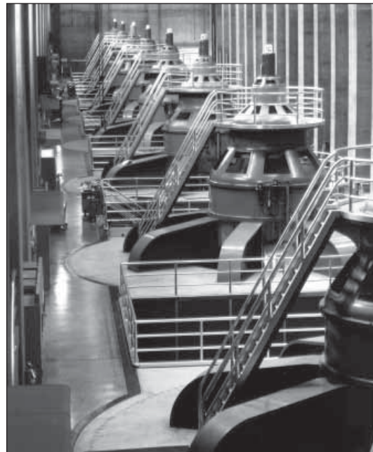
18.2. The interior of Nevada Powerplant at Hoover Dam.
