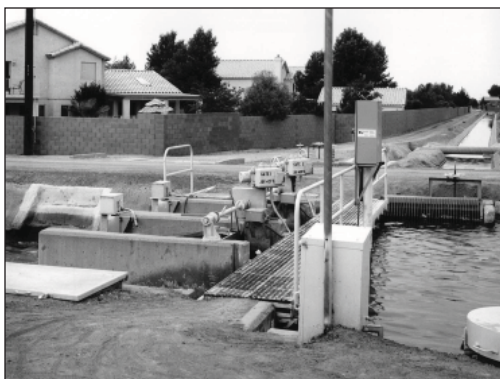
10.9. The SCADA system on the Salt River Project controls this canal control structure. Courtesy of the Salt River Project.
