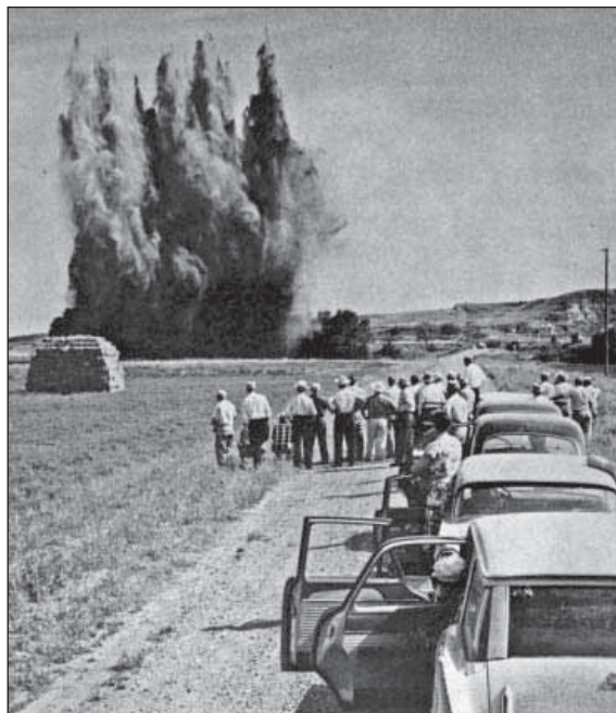
4.4. About 1959 Reclamation experimented with using dynamite to clean drains on the Lower Yellowstone Project.
