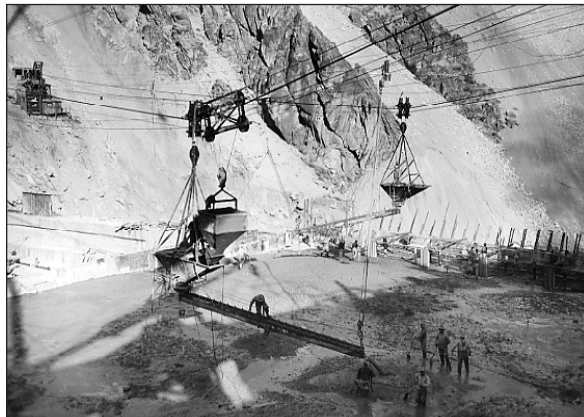
3.4. “Chuting” of concrete resulted in poor quality concrete.
