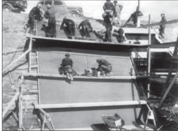
32.2. CCC crew placing and finishing concrete at a new Kingman check on the Owyhee Project in 1940.
