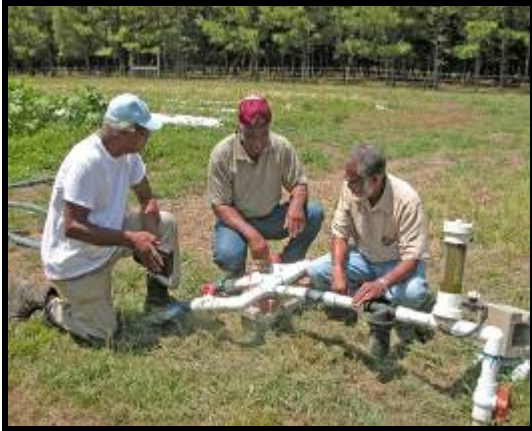
TSP/Eugene Hall, (left) talks with a producer about the installation of drip irrigation for a plasticulture system.
