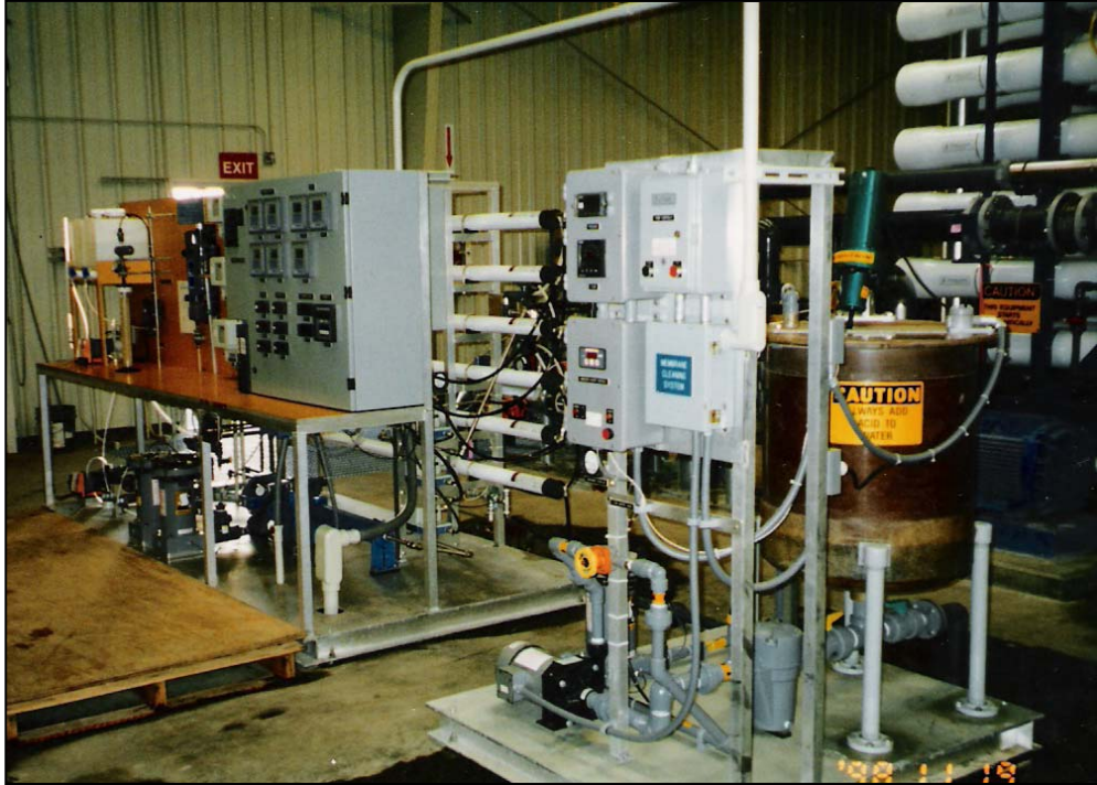
Figure 10. Cleaning Skid with Mix Tank, Heater, Circulation Pump, Cartridge Filter, and Instrumentation.
