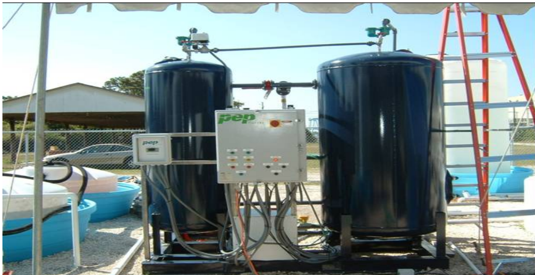
Figure 3-7. MMF Pretreatment Equipment Photograph.
