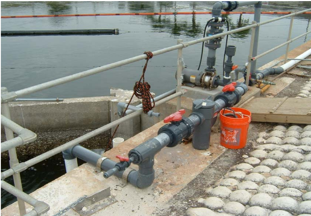
Figure 3-5. Seawater Intake Photograph.
