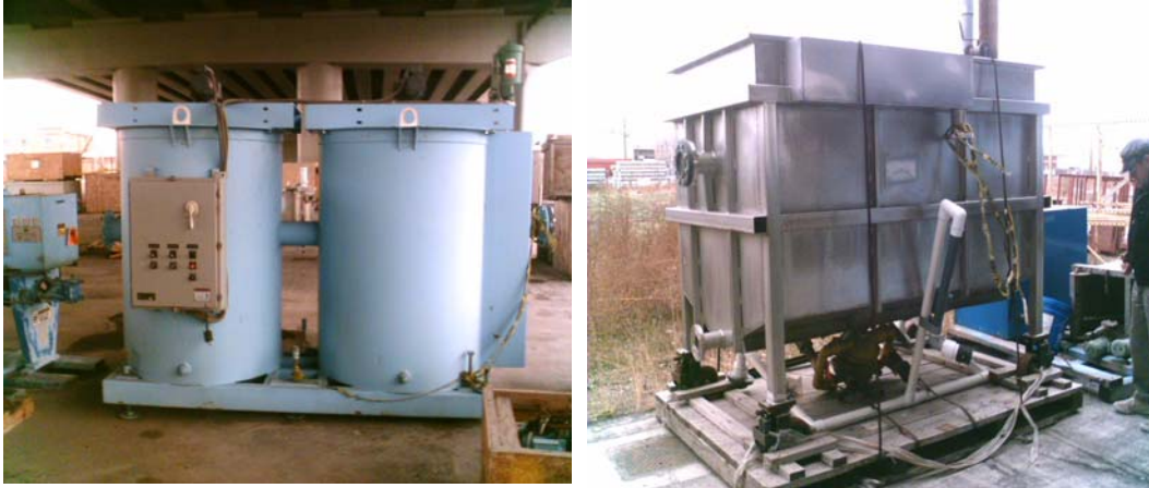
Figure 3-9. CSF - Flash Mixer/Flocculation Tanks and Parkson™ Lamella Plate Settlers.
