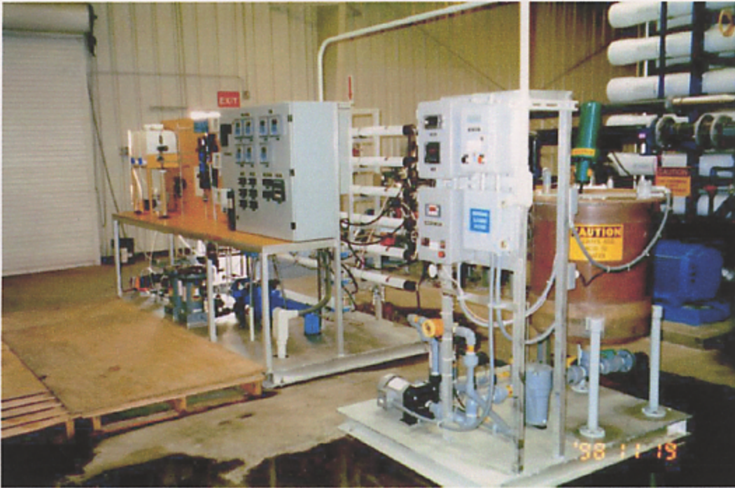
Figure 2.7. Membrane Test Bench (Front View)
