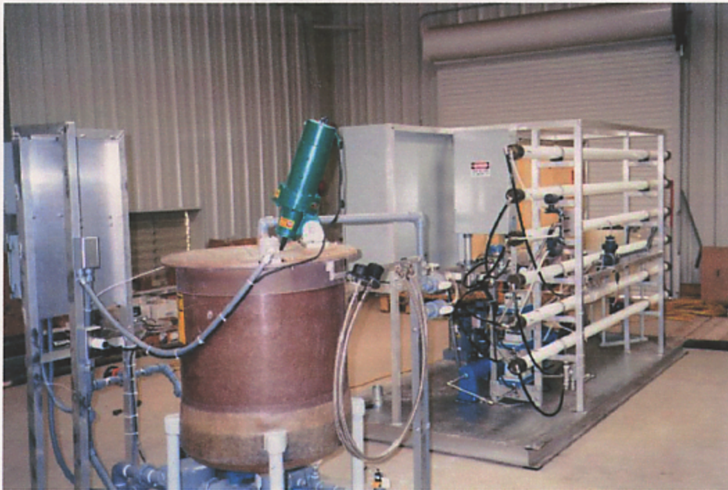
Figure 2.8. Membrane Test Bench (Rear View)
