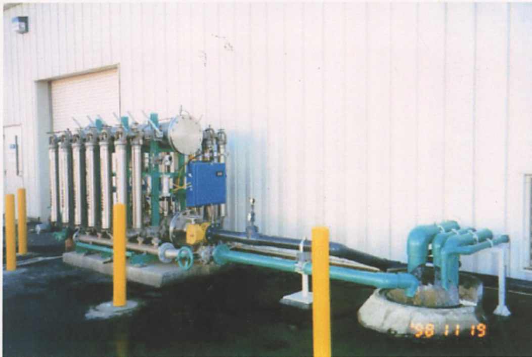
Figure 2.2. Automatic Backwash Bag Filtration System
