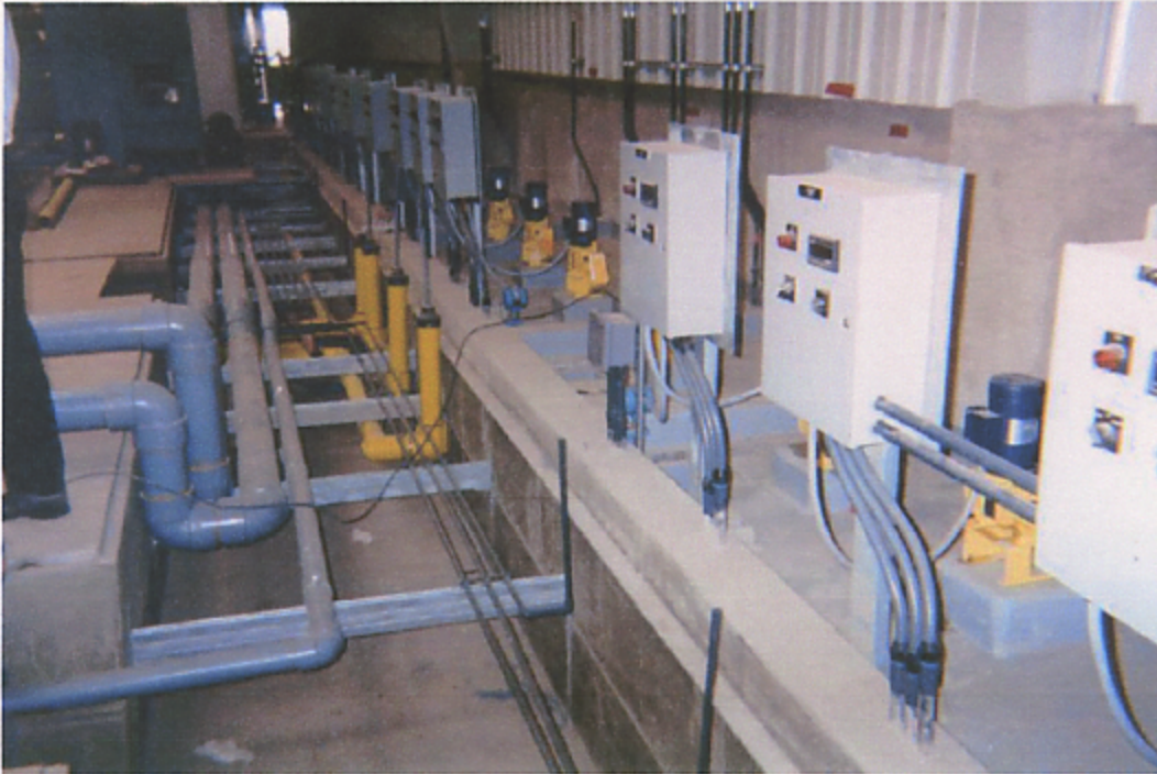
Figure 2.3. Chemical Metering Pumps and Controls.
