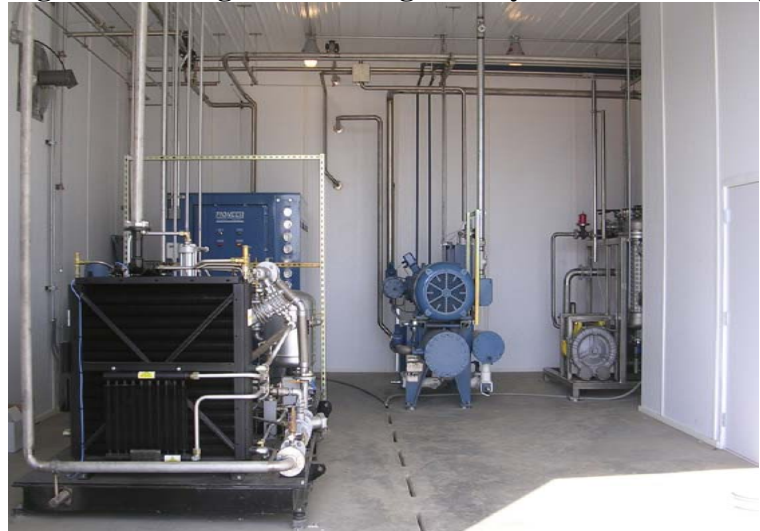
Figure 21 – Biogas Processing Facility at Emerald Dairy
