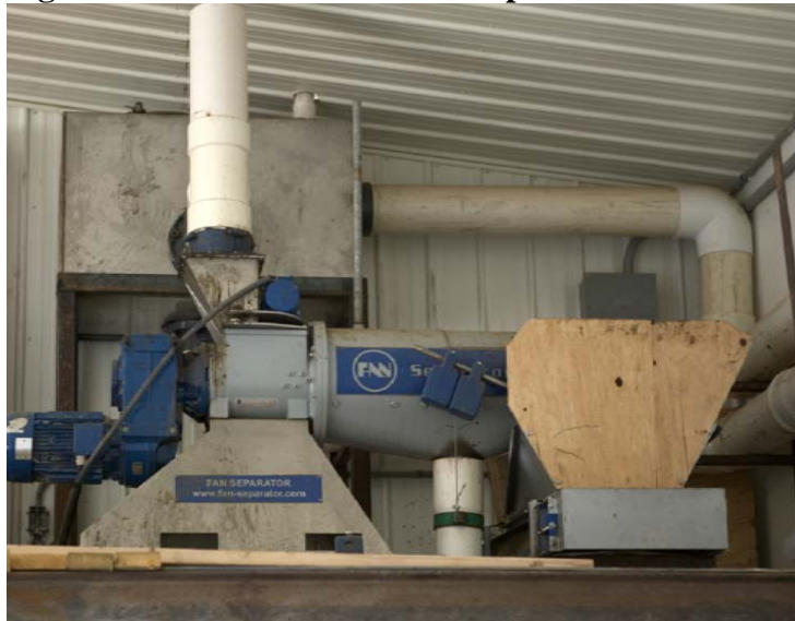
Figure 40 – Screw Press Solids Separator
