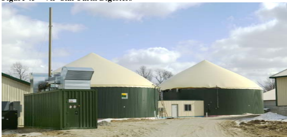
Figure 45 – Vir-Clar Farm Digesters
