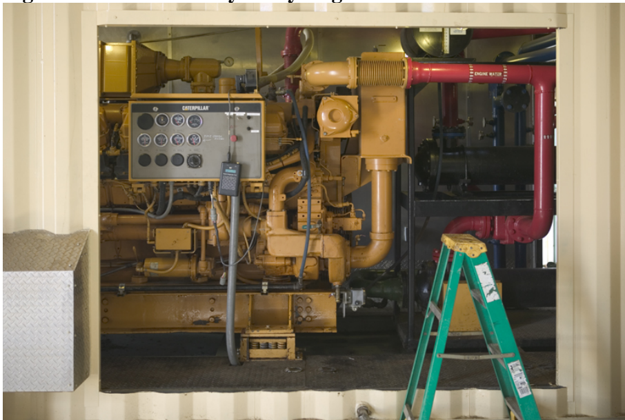
Figure 26 – Green Valley Dairy Engine Generator Set
