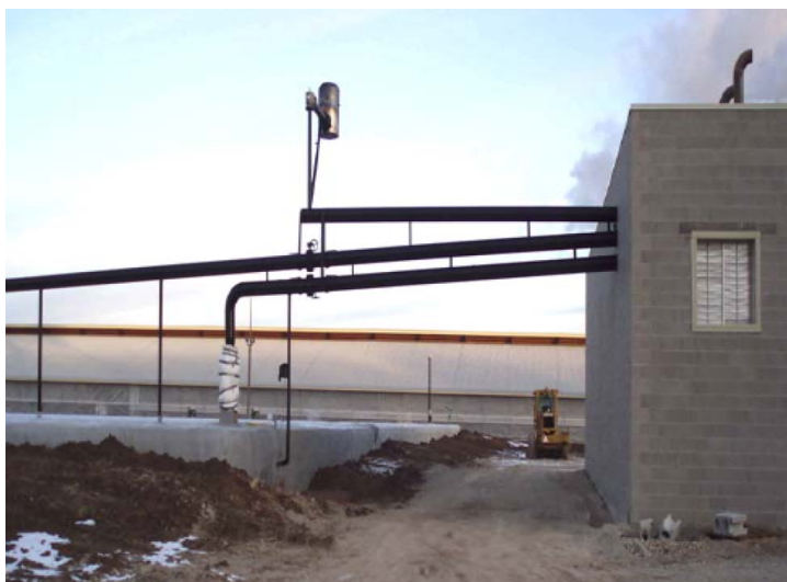
Figure 28 – Holsum Digester and Equipment Shed
