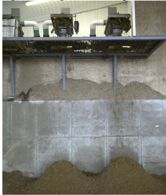
Figure 36 – Digested Solids Separation Area
