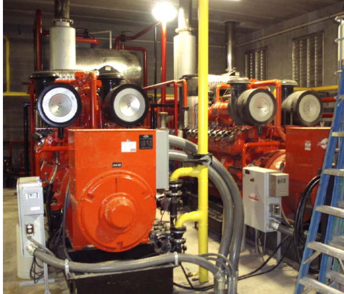
Figure 29 – Holsum Engine Generator Sets at Elm Road
