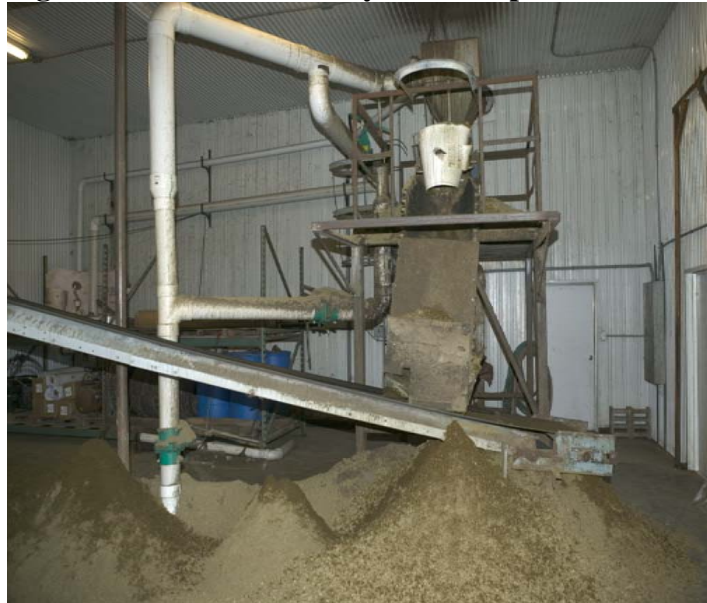
Figure 18 – Double S Dairy Solids Separator
