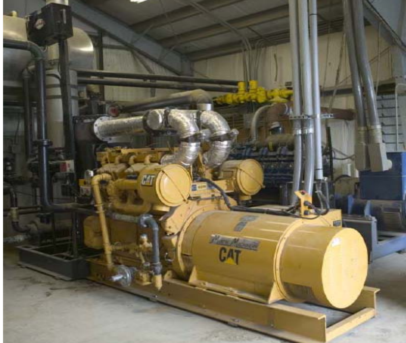
Figure 32 – Holsum Dairy Irish Road Engine Generator Set
