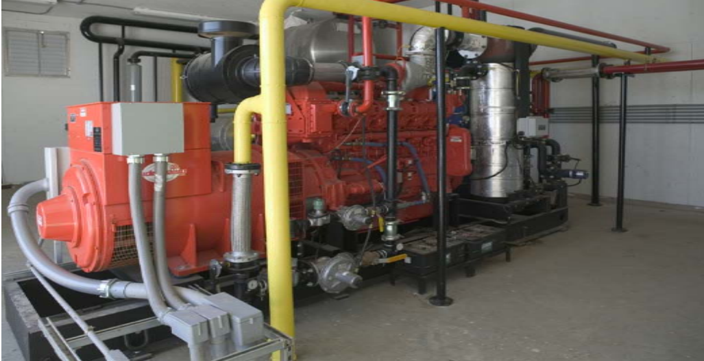
Figure 7 – Guascor 300 kW Engine Generator Set
