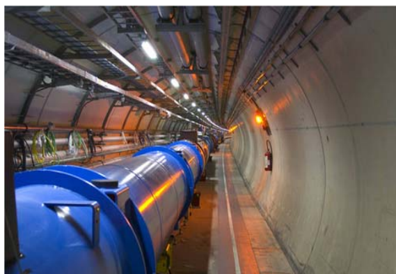
This is the underground tunnel of the Large Hadron Collider (LHC) accelerator ring, where the proton beams are steered in a circle by magnets. The LHC is the accelerator facility (in France and Switzerland) which will contain the ATLAS and CMS detectors. Credit: CERN ( www.atlas.ch/etours_accel/etours_accel01.html )
