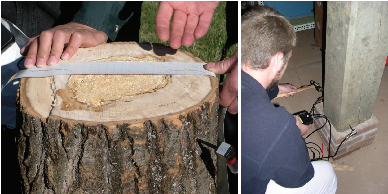
Fig. 49 & 50: Image B (left) shows the results of a resistance drilling test chart where a 3mm drill bit measures for wood density variations, note the paper as it measures density in a 1:1 ratio with the center or “rotten” portion of the stump showing as the dip in the readings. This device is not a truly a NDE tool it is minimally invasive to the point that it has little or no visual affect. Image 50 (right) shows the author using an impulse velocity tool which qualitatively determine areas of decay based on the transmission of waves through a wood. (Photo 49 by author and photo 50 by Danae Peckler, 2007)
