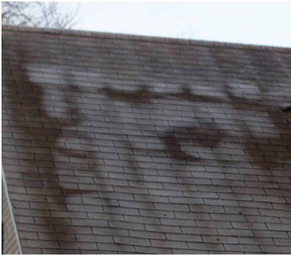
Fig. 9: A thermal bridge, such as the rafters in this photograph, act as a better thermal conductor than the surrounding materials, in this case fiber glass wool insulation. IRT can help make this differences visible without the need for a cold frosty morning. (Photo by author, 2007)
