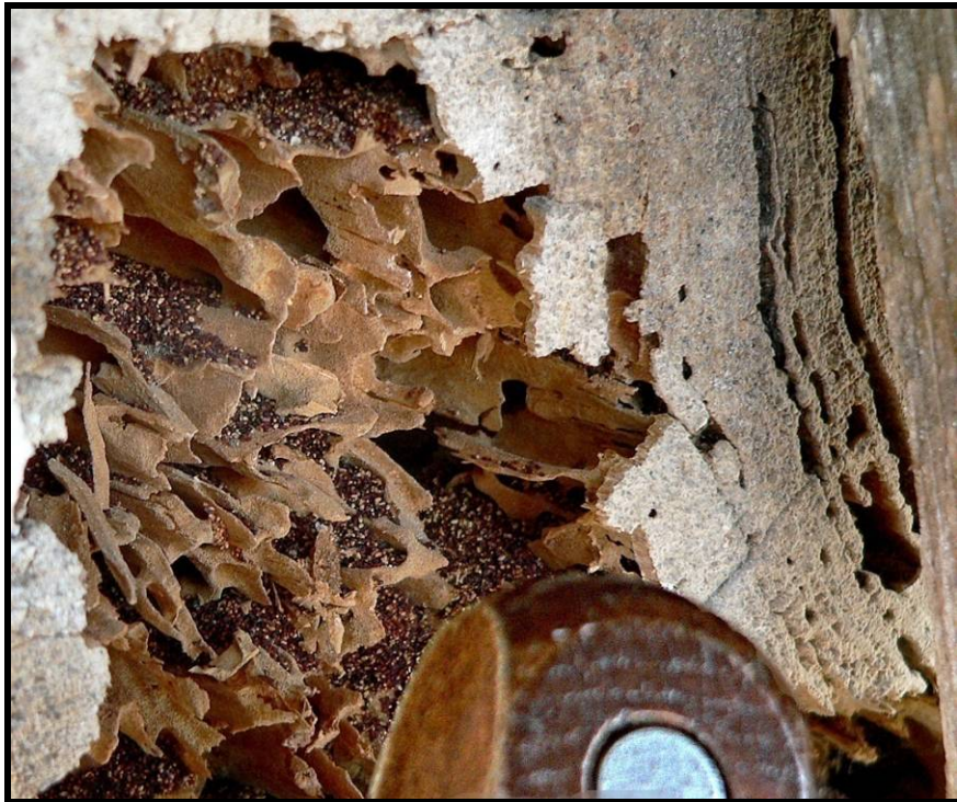
Figure 23. Typical drywood termite galleries discovered after breaking through a thin shell of sound-looking wood. Note the collection of fecal pellets.
