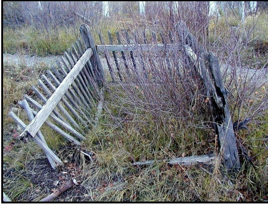
Figure 29. A grave enclosure damaged by decay and overgrowth of an invasive shrub in combination with decay of the corner posts.
