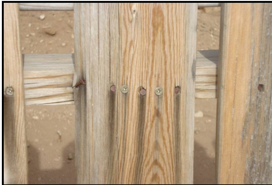
Figure 7. Stains on a grave enclosure caused by the combination of moisture and a chemical reaction between extractives in the wood and the metal fasteners.
