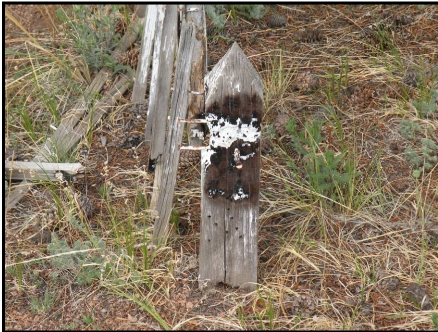
Figure 28. A grave enclosure corner post damaged by fire.
