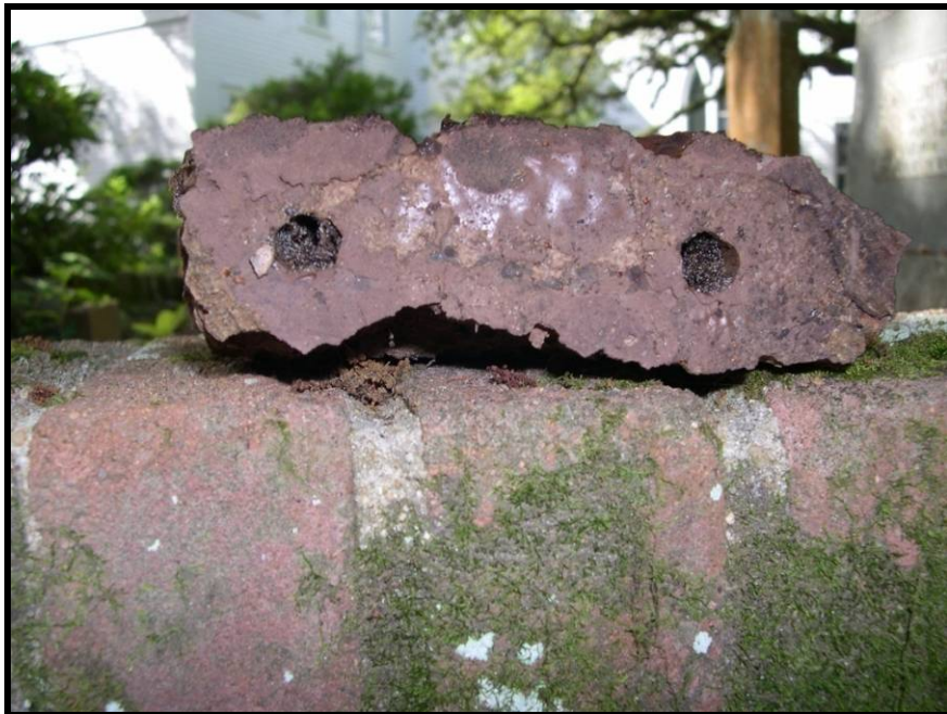
Figure 46. The repaired end of the marker (from Figures 43, 44, and 45) shows that the epoxy is in good condition but the wooden dowels have rotted away.
