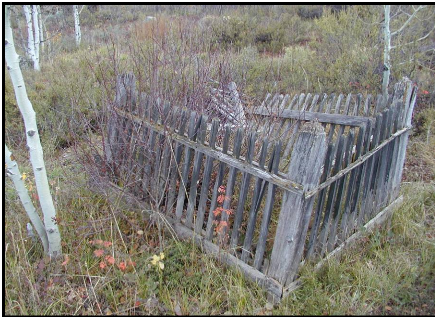
Figure 19. A grave enclosure in partial collapse due, in part, to decay of the corner posts at ground level.
