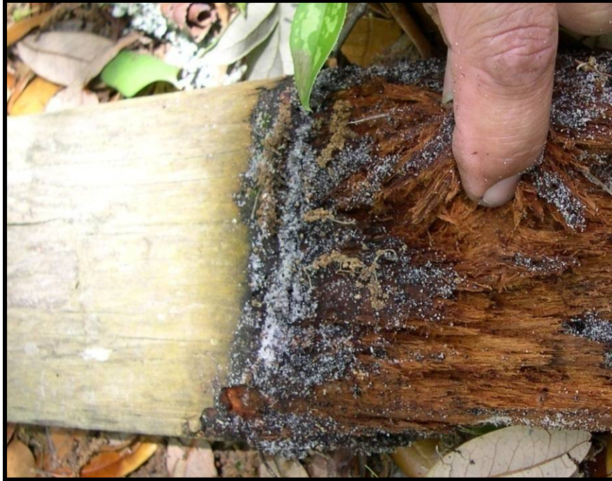
Figure 18. Evidence of advanced decay – the wood is soft and easily breaks apart.
