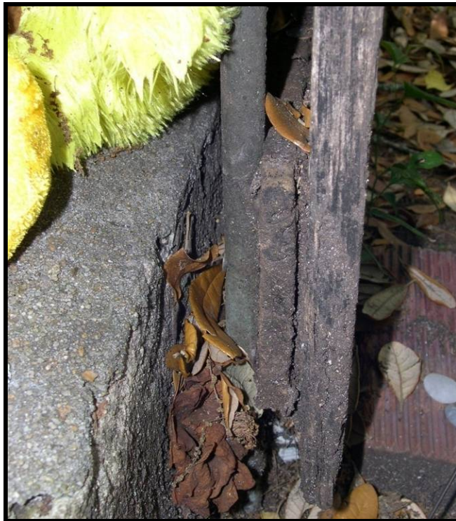
Figure 51. A close-up of the side view of the repair showing the wood the marker has been sandwiched to and the copper pipe, along with organic debris.
