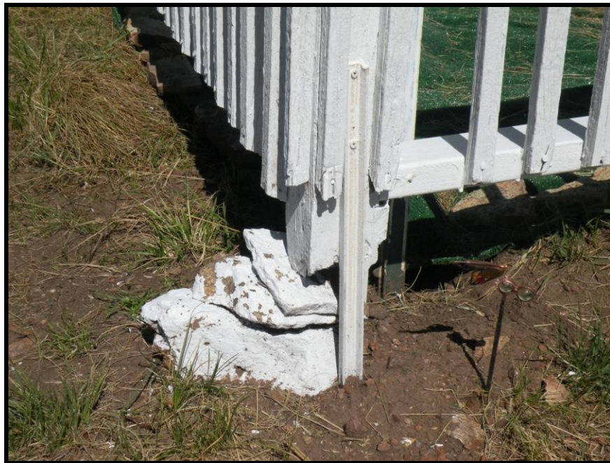
Figure 52. The deteriorated base of a grave enclosure corner post has been replaced by a channeled metal rod and natural stones, painted white.
