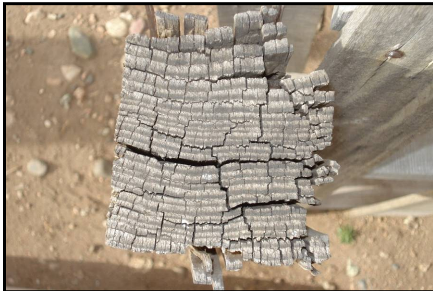
Figure 2. The top of a grave enclosure corner post showing splits developing from cyclic moisture or freeze/thaw episodes.
