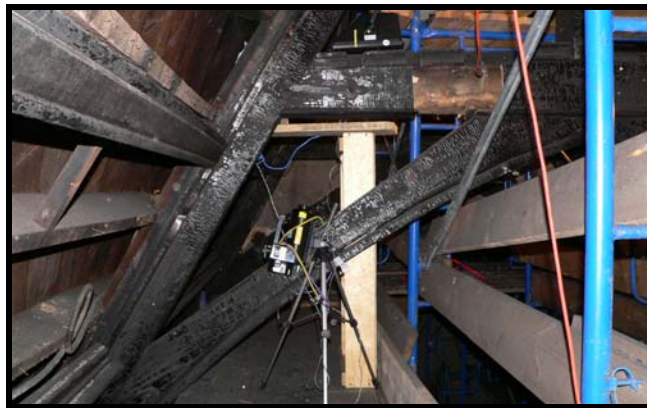
Figure 100. Source and imager placement to view the bolt through the tie at Location B1 on Truss 7 (north side).
