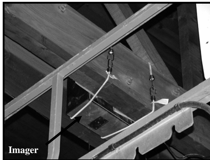
Figure 9. Imager attached to repaired bottom truss chord.
