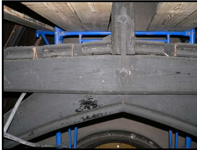
Figure 102. Area of interest showing two bolts and a metal strap at Location B2 on Truss 6.
