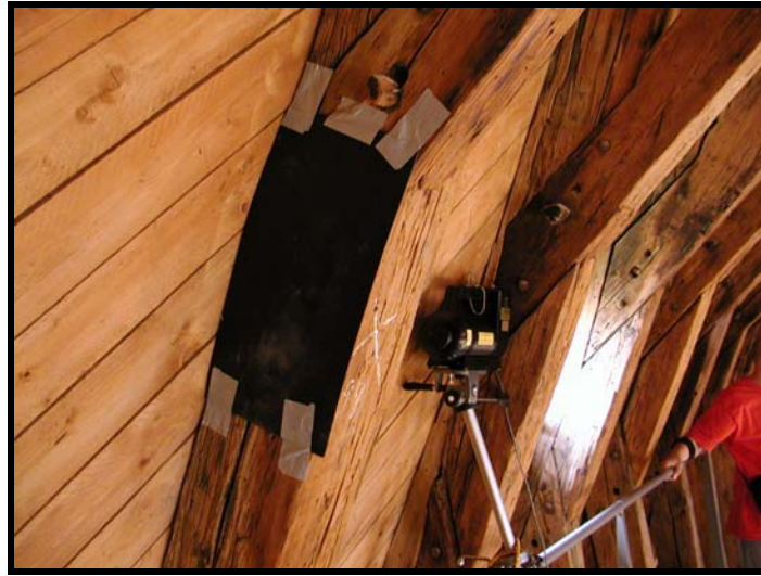
Figure 92. Test configuration for digital radiography of a roof truss member in Saint Anne's Church.
