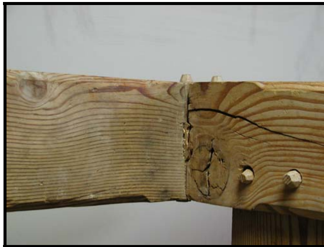
Figure 36. Mortise and tenon joint viewed at an angle from below the joint.
