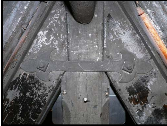
Figure 106. Area of interest showing two bolts and a metal strap at location A on Truss 7.
