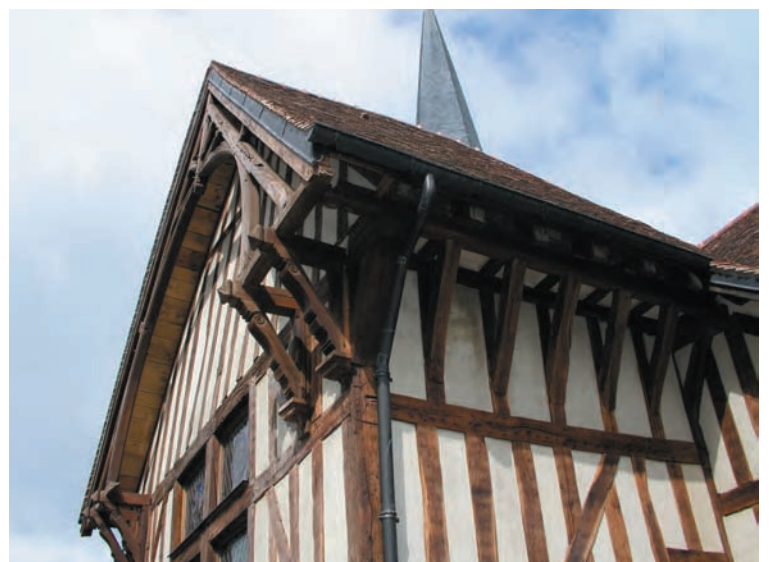
Church of St. Julien and St. Blaise, Longsols, originally 15th century, recently restored. The framed gable end overhang with carved double brackets and arch braces shows the possibilities of the framer's art before structure and decoration were disconnected by the Renaissance. Interior shown overleaf.
