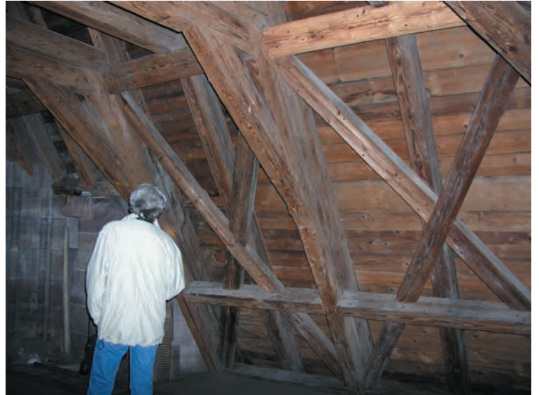
Softwood Liegendestuhl (lying chair) trusses and heavy longitudinal X-bracing support the framing of the weather roof of Strasbourg Cathedral. Such German-style framing prevails in Alsace.
