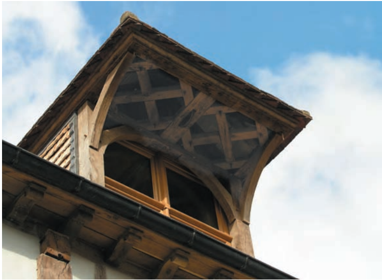
Substantial dormer at Troyes, so heavily framed perhaps to support loads brought up on the pulley just visible at the center of the overhang. Lead flashing shields the thick edge of the tile siding.
