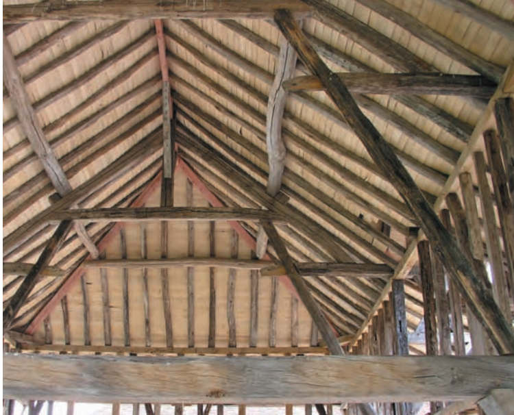
Newly framed structure, Montreuil, using old and new timbers, the latter painted for yet more contrast. Note legs of strength to carry roof loads down from collars to tie beams, thus dissipating much rafter action.
