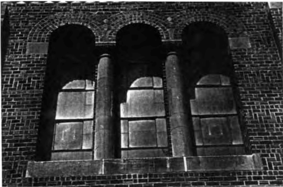
Fig. 26. Due to cloudy PG, these windows no longer read as apertures in the wall.
