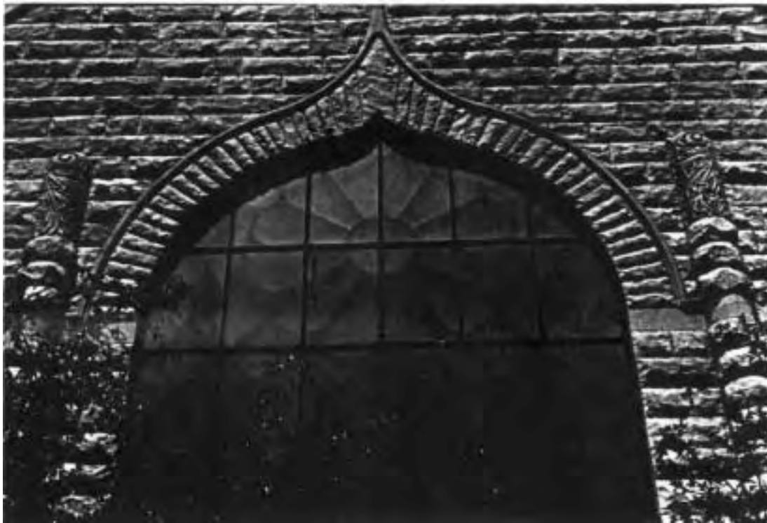
Fig 29. Another PG installation on the same building disregards the tracery.
