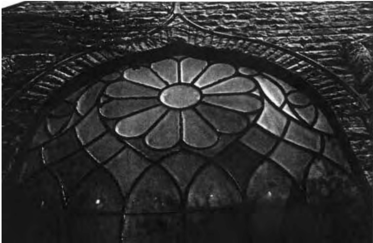
Fig 28. This PG needs maintenance, but the muntins conform to the tracery.
