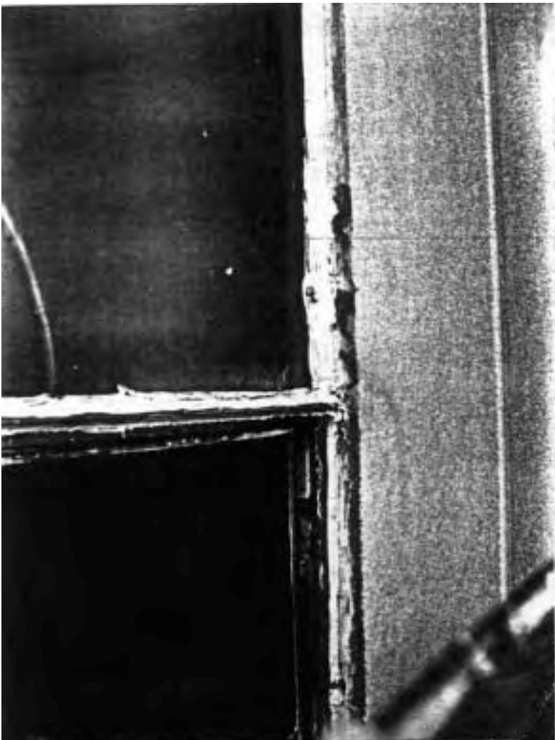
Sealants had been applied poorly on the existing PG.
