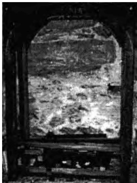
Figure 8: View of the Wall Construction behind The Facade From the Interior Stone Rubble and Lime Mortar
