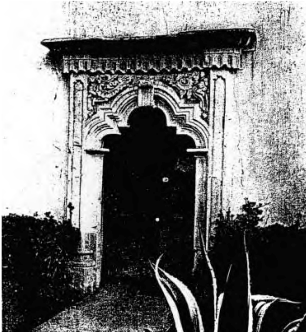
Figure 15: A copy of a 1934 HABS photograph of the west transept doorway shows some areas of decay that have subsequently been repaired.
