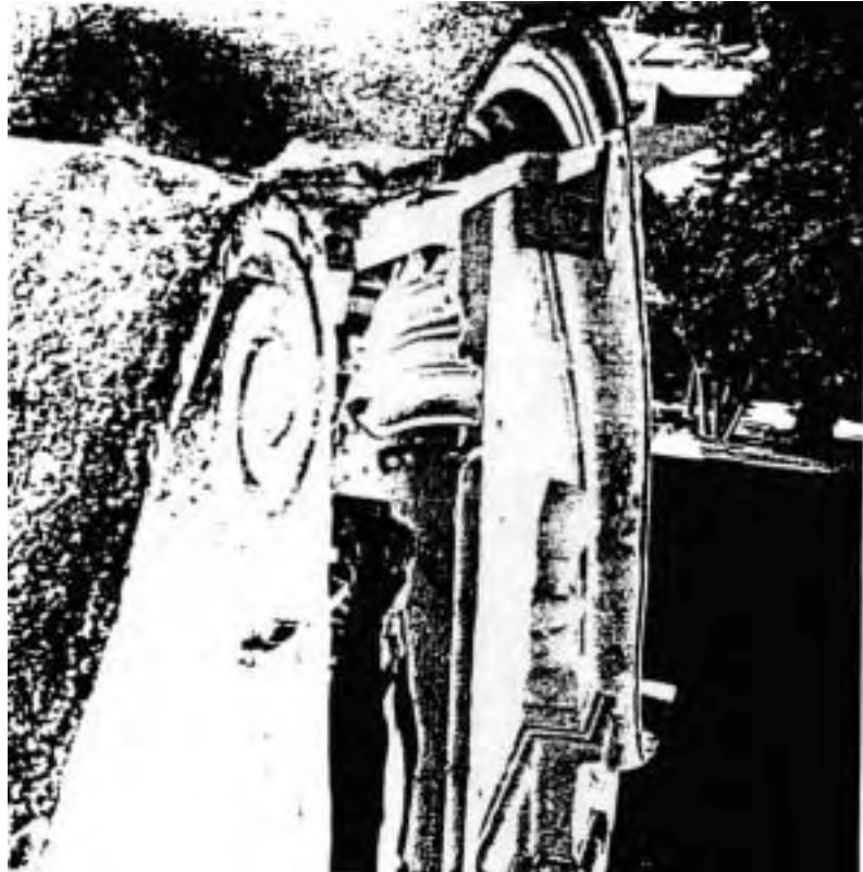
Figure 11: An oblique view of the upper part of the facade and the juncture of the volute and the parapet cap. Note the rust and gold lichen at the interface.
