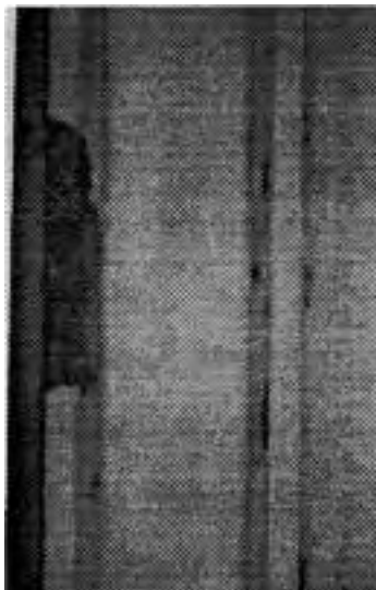
Figure 6: Spalling of Cement Repair
