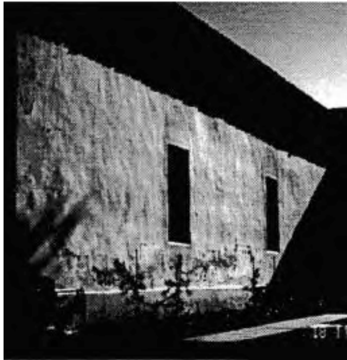
Figure 3: Water Damage (runoff, wind driven rain, and rising damp)
