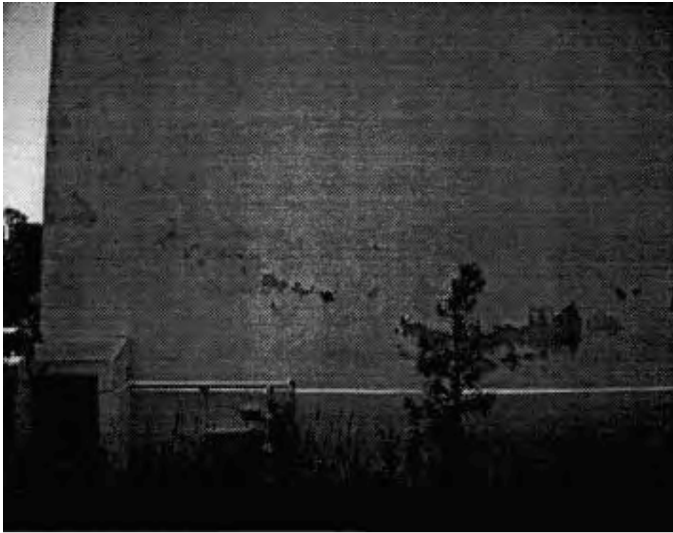
Figure 2: Tideline on West Wall
