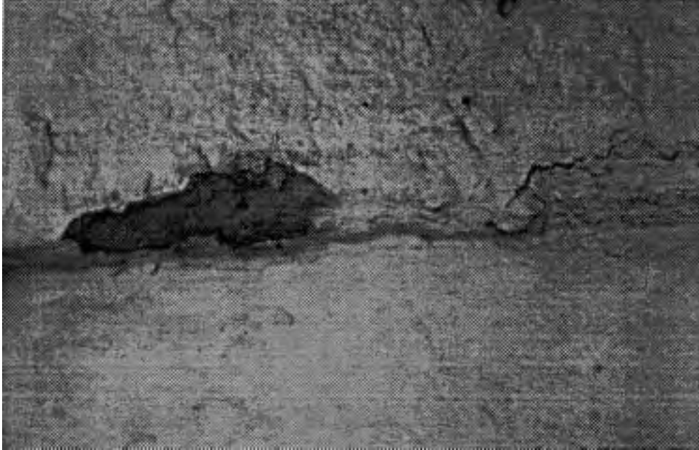
Figure 5: Spalling of Cement Patch adjacent to Lime Based Rendering
