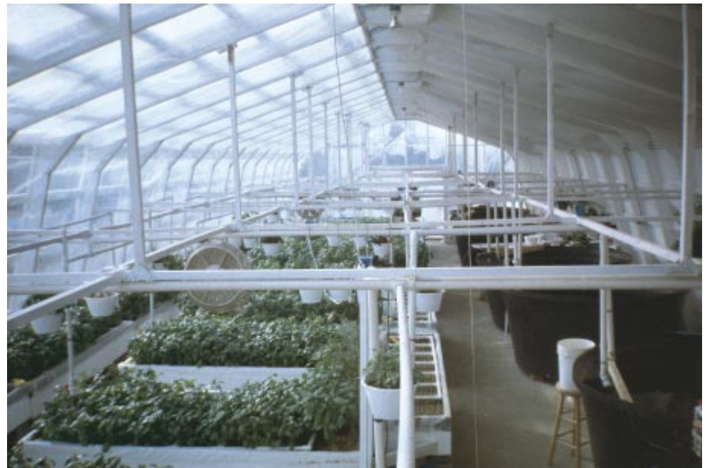
All the plumbing that links plant beds to fish tanks is overhead in the Speraneos' system.
