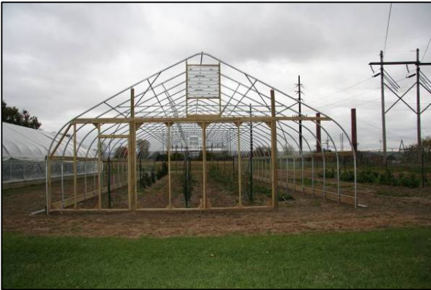
Figure 13. Peak-style high tunnel framing – front view shows end framing. Doors open outwards at both ends.
