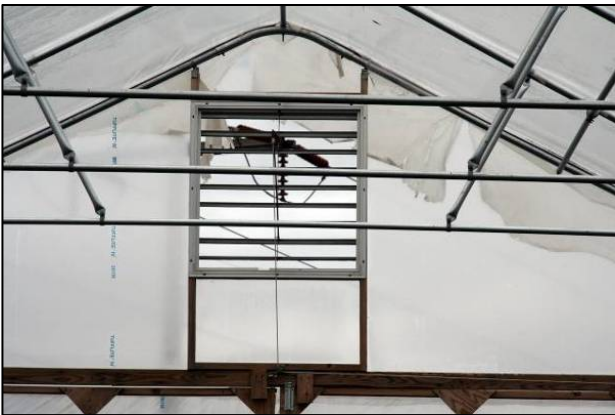
Figure 26. Venting the tunnel – peak vents.
