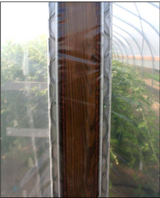
Figure 18. Fastening the plastic to batten boards with wiggle wire. The wire secures the plastic by pinching it in a channel.
