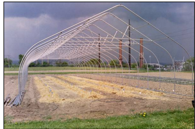
Figure 8. Peak-style high tunnel ribs (bows).
