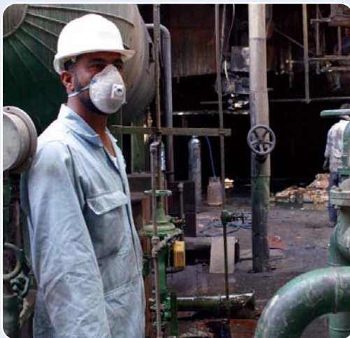
Iraqi workers carry out renovation of the Al-Doura power plant in Baghdad, Iraq. USAID is funding the repair of Iraq's nationwide electrical system.
