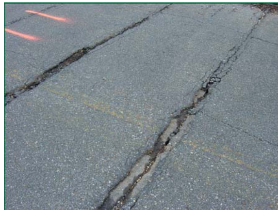
Figure 2. Transverse cracks in the asphalt wearing surface at panel joints.
