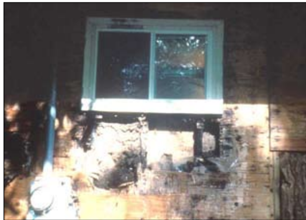
Alternative methods of installation will be investigated to help avoid improper installation as seen above. Moisture intrusion can and will lead to decay in wood associated with windows.
