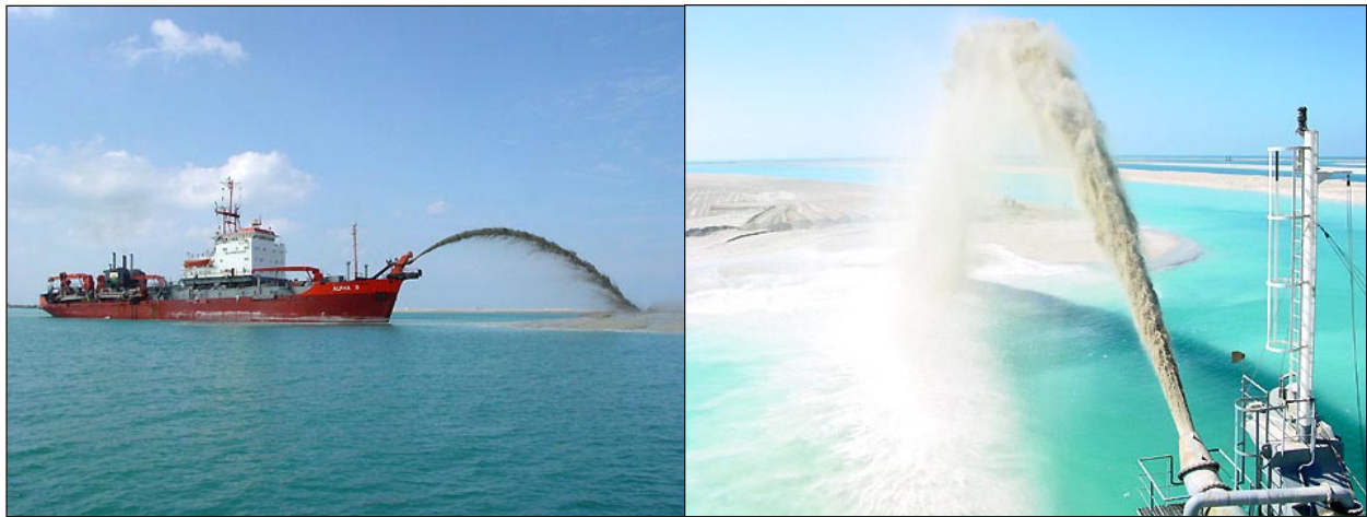
Figure 8. Dredgers throwing sand into a nourishment restoration project. Photo courtesy of Bert Visser's Directory of Dredgers. http://www.dredgers.nl
