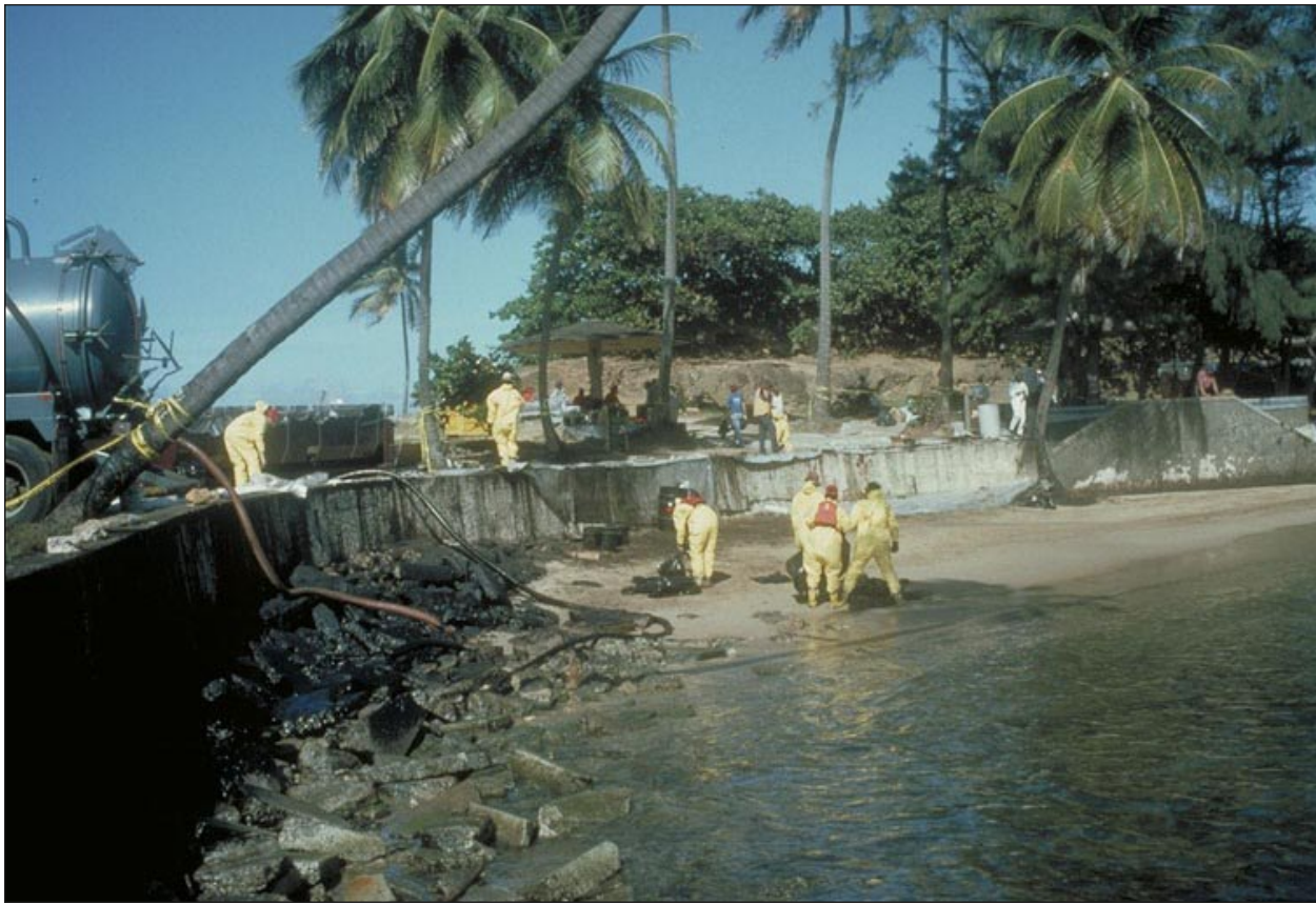
Figure 4. Cleanup workers use vacuums to remove oil from rocky shores of San Juan, Puerto Rico. Photo courtesy of Morris Berman. NOAA Office of Response and Restoration (ORR) photo gallery.
