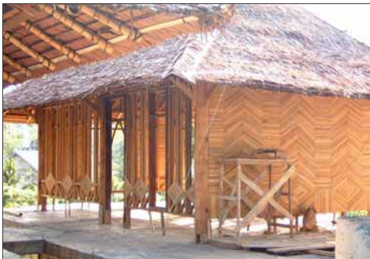
Figure 4. Community houses in Indonesia using wood of mangrove trees. Photo courtesy of the Mangrove Action Project, Port Angeles, WA 98362-0279 USA. http://www.earthisland.org/map/mngim.htm
