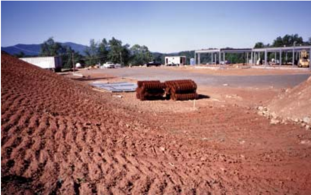
Figure 17. —A construction site on a sloping landscape. Sloping landscapes often have cut and fill areas that can be used to make building sites more level. Soils information for building site development is useful for planning and site design.
