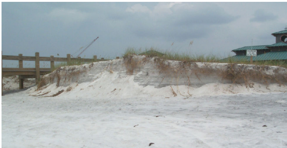
Dune front at Ft. Walton Beach, FL, lost during Hurricane Ivan in 2005. The buildings were not damaged.
