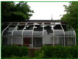
Lean-to greenhouse destroyed
