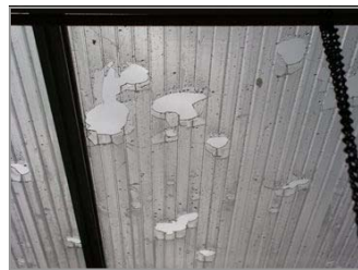
Main greenhouse roof damage close-up
