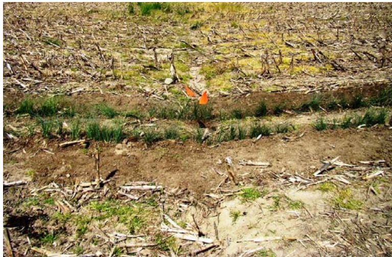
Figure 3. Trench backfilled with soil excavated by trencher. Finished barrier in place and functional.
