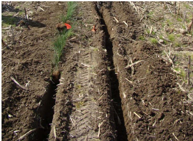
Figure 2. Installing vegetative sod strips in trench. Note: Vegetative sod strip spans concentrated flow area.
